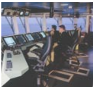
An example of a UNIMACS 3000 bridge for a navy vessel, produced by Imtech Marine & Offshore, Rotterdam.
